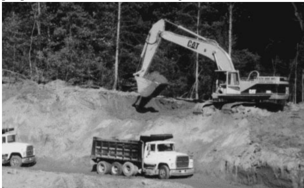
Figure 1. Excavator loading a truck with soil in a typical mass excavation work scenario.
