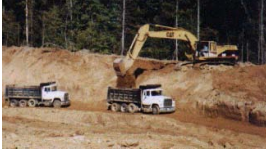
Figure 19 Excavator loading a truck in a mass excavation scenario. The excavator sits on top of an elevated bench, removes the material from the bench, and deposits it into the back of the truck.
